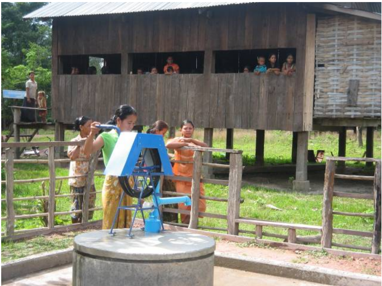
Installed Rovai pump at the meeting hall in Vorng
